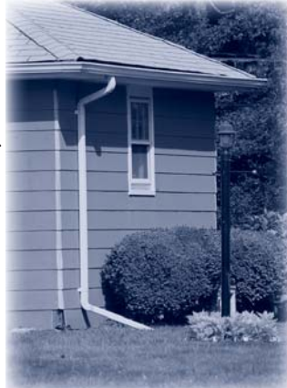
A well-placed downspout directs stormwater onto permeable ground. Photo by Rory MacNish, CCE.
